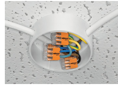
Lighting distribution in a ceiling canopy
